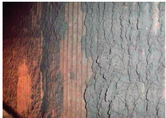
Figure 6 - Slag formation on boiler tub
