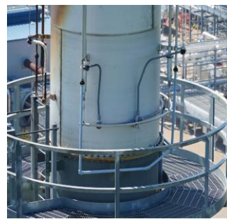
Pilot #1 and #3 Manifold/Conduit
