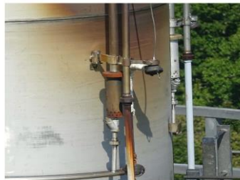
View of Pilot Gas Mixer #3 (225 Degrees) (1" Pilot on the left of the ladder)
