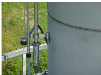
View of Pilot Gas Mixer #1 (45 Degrees) (immediate left facing utility piping)
