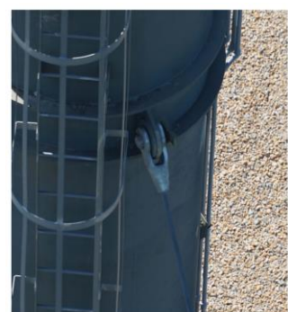
Gas wire Stack Connection #1 (90 Degrees) (Closest to Ladder)
